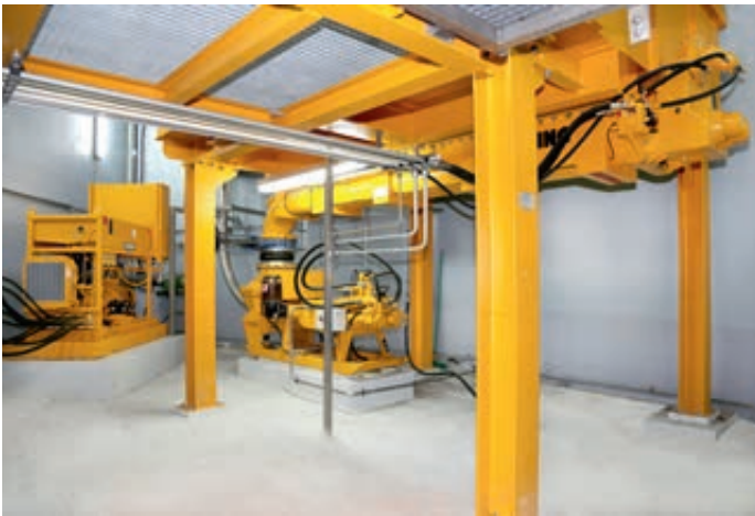
Pumping of dewatered sewage sludge in a waste water treatment plant Germany
