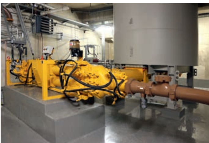
Pumping of dewatered sewage sludge in a waste water treatment plant Germany
