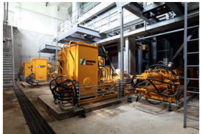
Pumping of dewatered sewage sludge in a waste water treatment plant China
