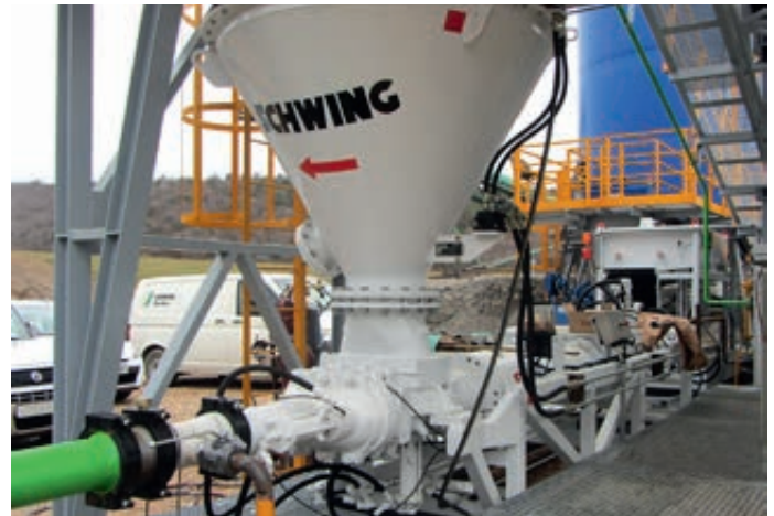
Pumping of fly ash in a power plant Croatia
