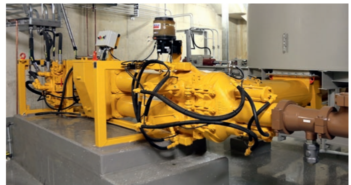
WWTP Buchenhofen, Wuppertal, Germany
